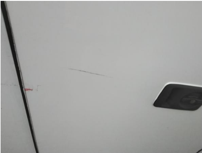
11: Door osr Dented With Paint Damage
